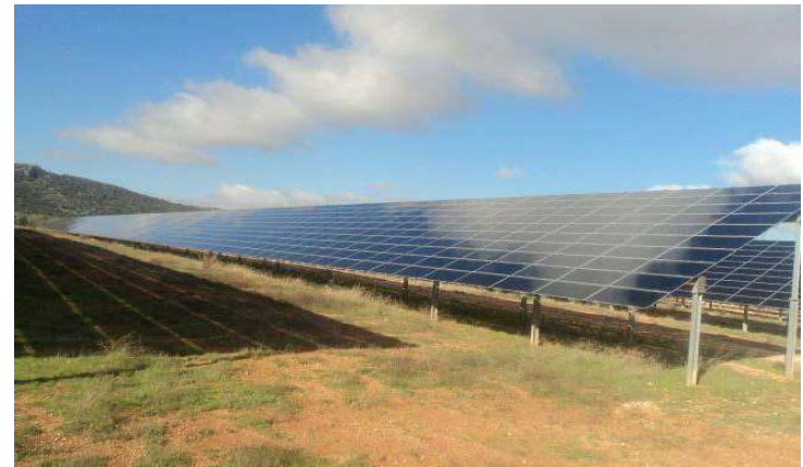
Lora solar PV plant (2 MW) located in Sevilla near the south coast of Spain
