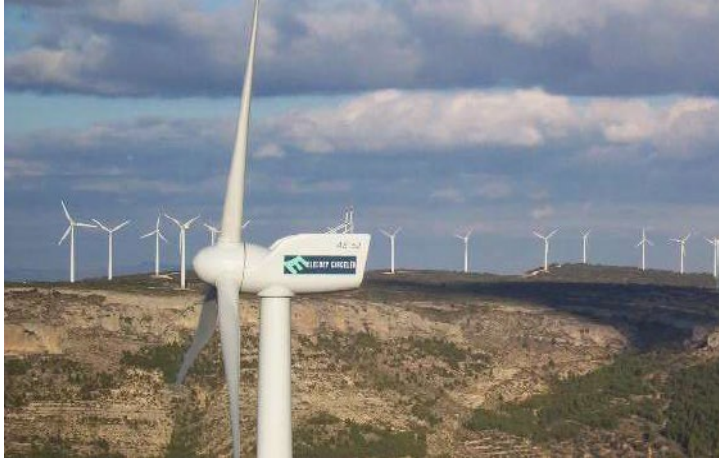
Carcelen wind farm (50 MW) located in Albacete (east coast of Spain, south of Madrid)
