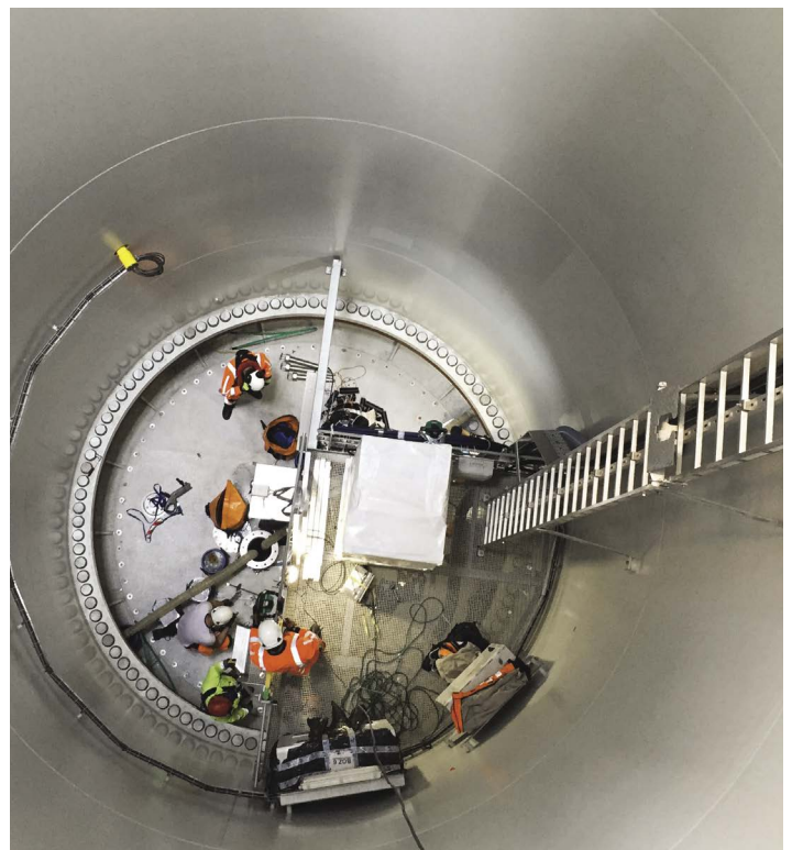
Transition piece assembly at our 600 MW Gemini offshore wind farm. Photo by Gemini Windpark
