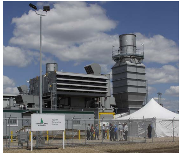
Our 86 MW natural gas facility, Spy Hill, in Esterhazy, Saskatchewan uses turbine technology to produce electricity in an efficient, reliable and environmentally responsible manner.
